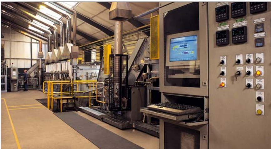
New InTouch controlled furnace
