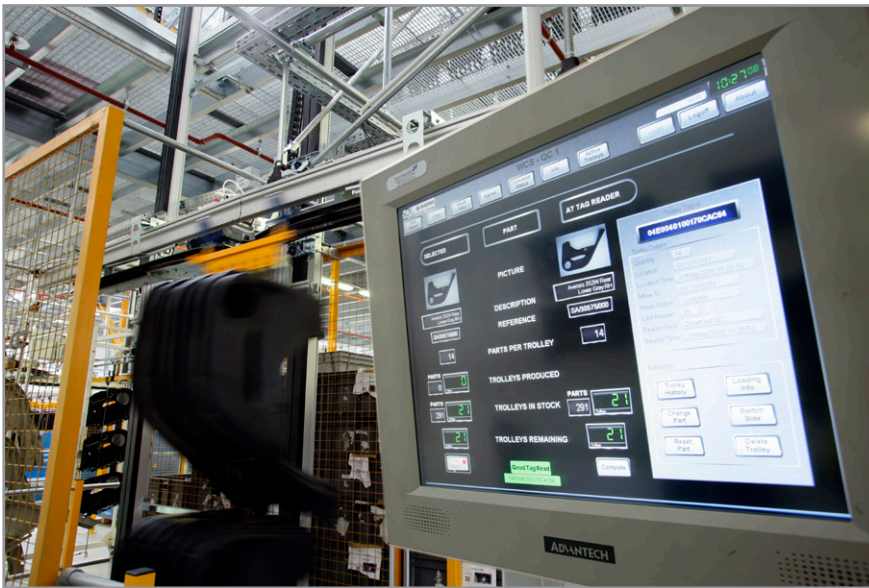
Operator Station with Touch Screen PC
