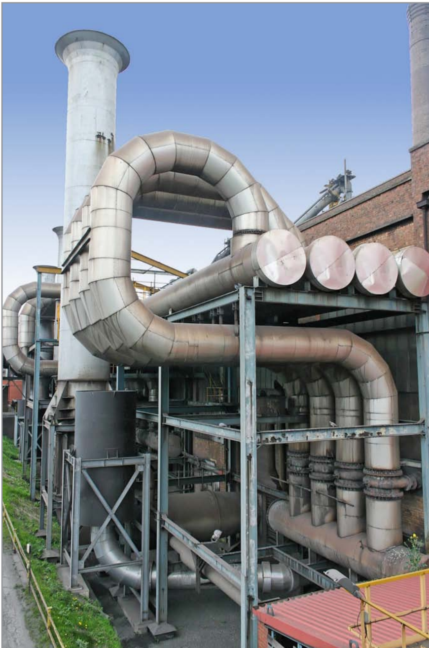
Air intake and Blast manifold
